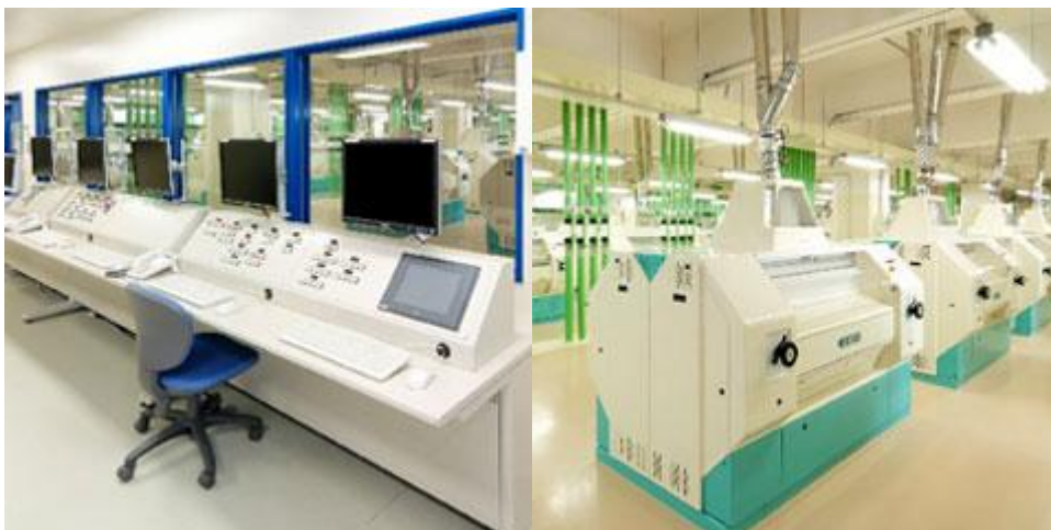
▲ Central Control Room
